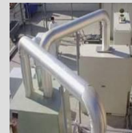
UTC Power: Power systems, fuel cells
